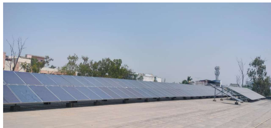
PV Panel on Administrative Building Rooftop
